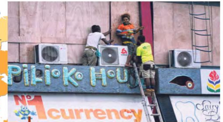
Locals in Vanuatu boarding up their shops in preparation for Cyclone Harold on April 6. This is to prevent their windows from breaking and water flooding the building.
